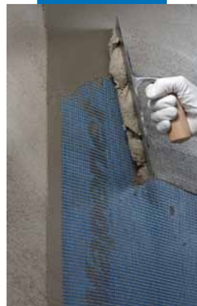
Application of the second layer of Planitop 200 on a substrate made from different materials with Mapenet 150 embedded between the layers
