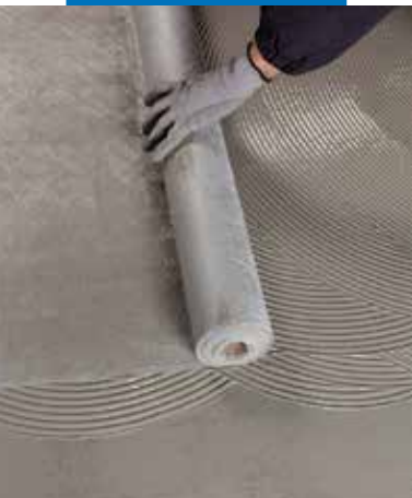
Placing Mapenet Sel on the first layer of Mapelastic Turbo while wet
