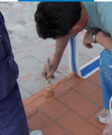
Waterproofing a distribution joint with Mapeband fixed in place with Aquaflex Roof
