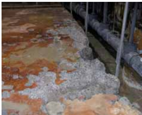
Deteriorated concrete due to chemical attack
