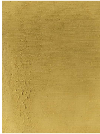
Example of 'mud cracking' when substrate hasn't been correctly 'damped down' or limewash dilution rates are not correctly observed
