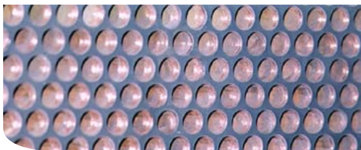
Condenser Tube Sheet Repaired with Scotchkote Epoxy Metal Repair EG 503 and refurbished with Scotchkote Epoxy Ceramic Surfacers FG 512.
